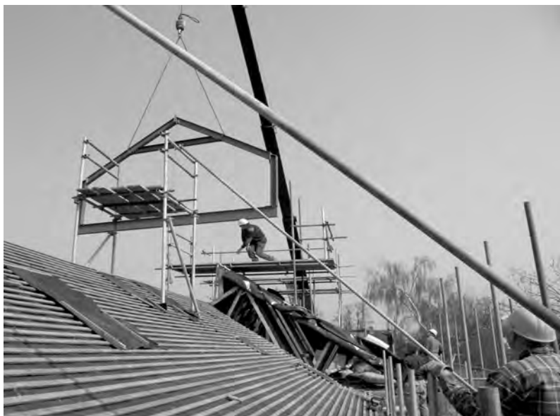
Mayfair in April – the builders begin to strip the roof and a giant crane swings into place the steel frames for the second storey.
